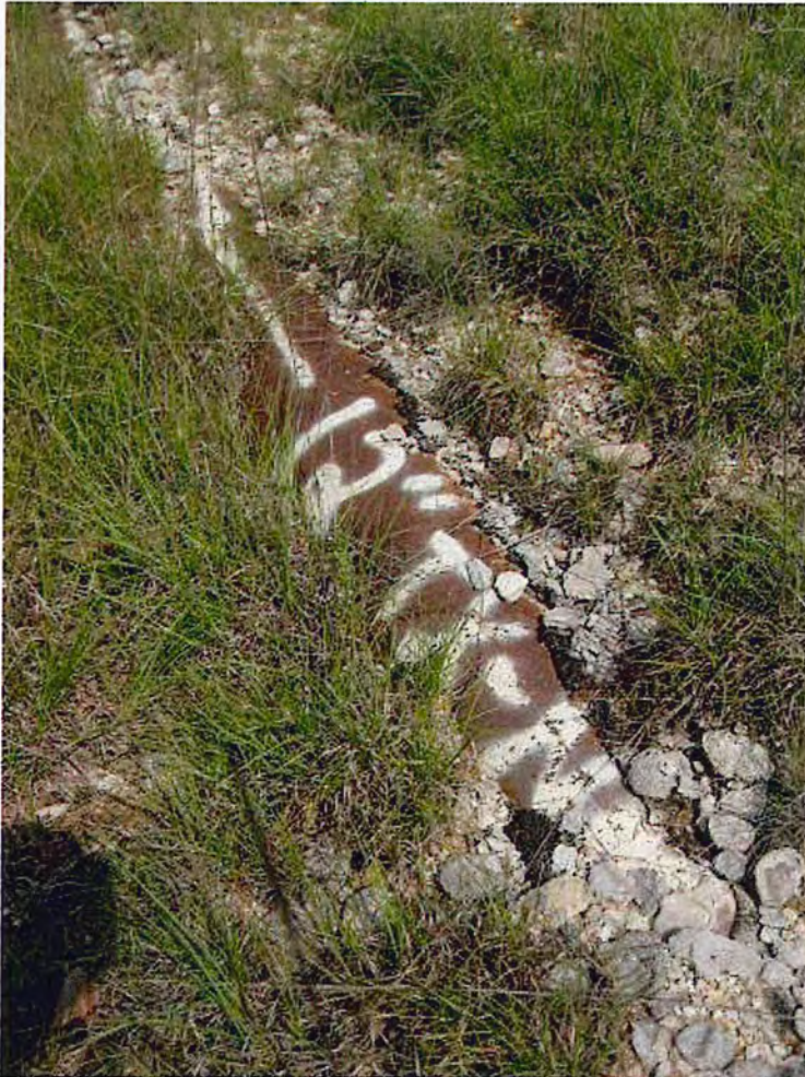
Photo 1. Exposed gas pipeline
